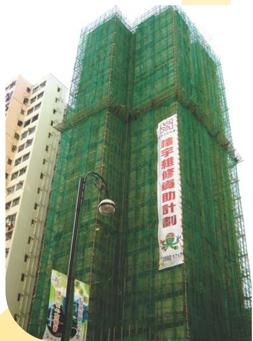
獲房協資助進行維修工程的樓宇 Building undergoing maintenance with the assistance of Housing Society
