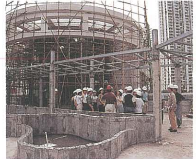
各準業主在房協代表帶領下參觀雅景臺地盤，從而了解工程進度 Purchasers-designate gained first-hand information on the progress of construction in a visit to the Park Belvedere site
