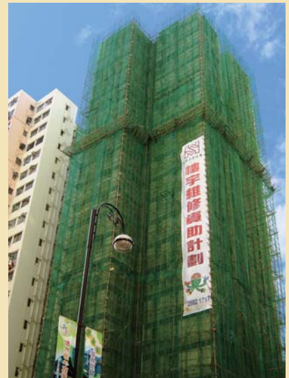
A building carrying out maintenance work under BMMS 資助舊樓進行大廈維修工程
