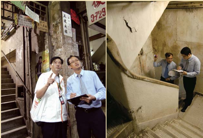
PMAC staff inspecting buildings in the old districts 「物業管理諮詢中心」職員在舊區勘察樓宇狀況
