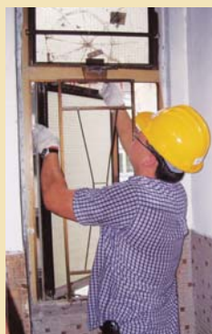
Free window inspections are offered to private buildings in Hong Kong 為私人樓宇提供免費鋁窗檢查服務
