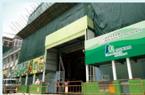
Demolition work underway at the Po On Road / Wai Wai Road project site in Sham Shui Po 深水埗保安道／懷惠道市建項目地盤進行拆卸工程
