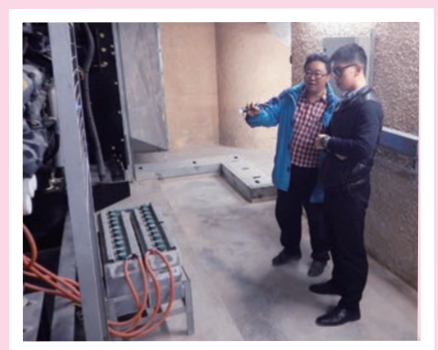
梁同學(右)參與檢查「雋悅」的電力裝置系統 Leung (right) participated in the inspection of the electricity system at The Tanner Hill
